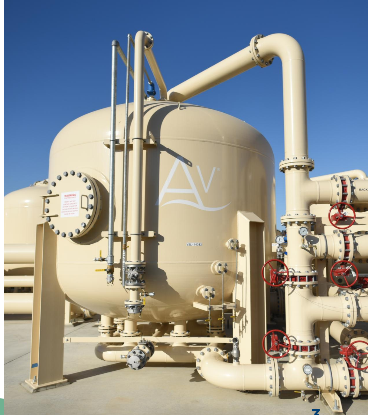
Stoneridge PFAS Treatment Facility
