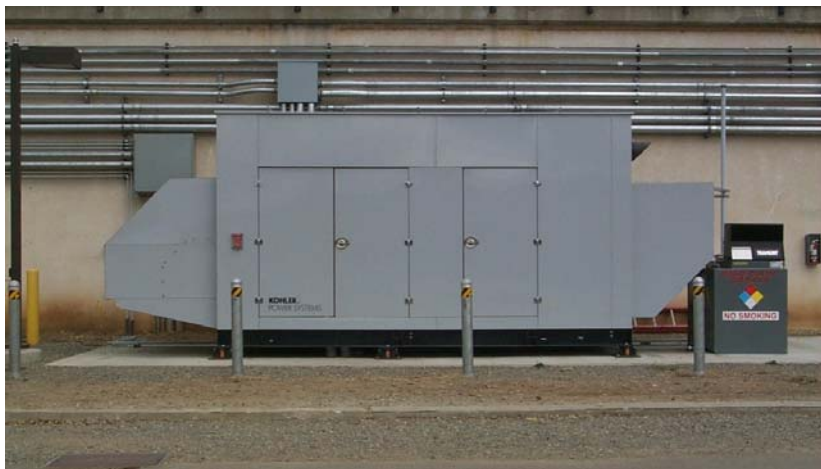
A new 500-kilowatt generator at the Del Valle Water Treatment Plant
