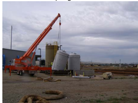
Crews replaced a 5,600-gallon ferric chloride tank with two new 8,000-gallon tanks at Patterson Pass Water Treatment Plant.
