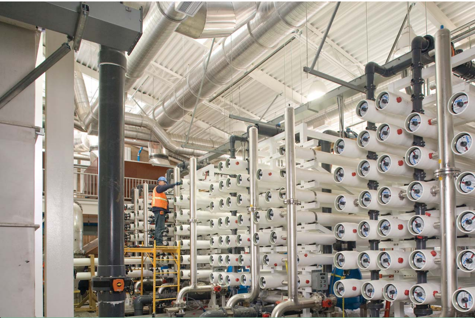
Mocho Groundwater Demineralization Plant Membrane Modules
