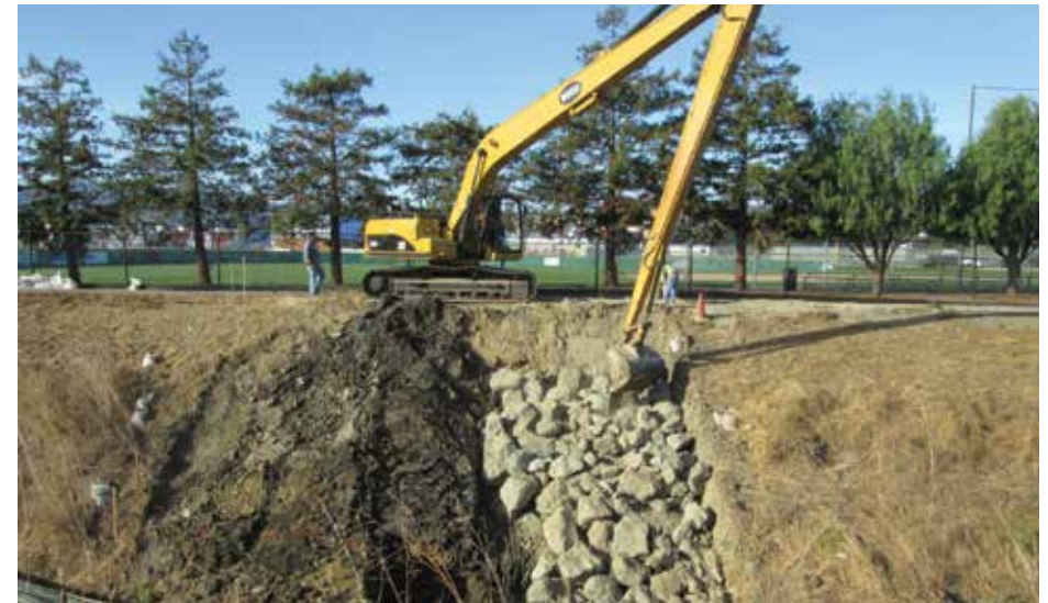
Slide repair along South San Ramon Creek in Dublin
