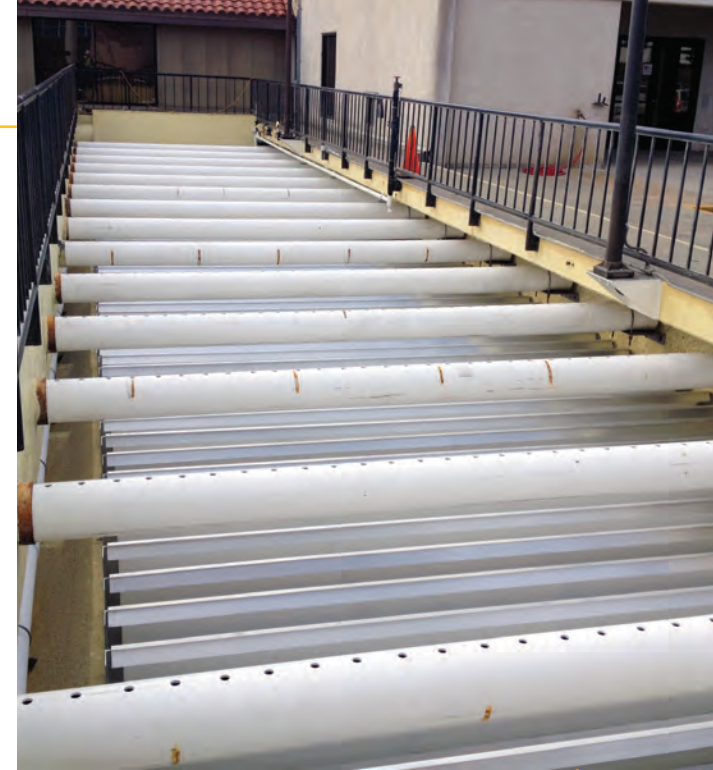
Phase 1 of the Superpulsator Rehabilitation Project at the Del Valle Water Treatment Plant was completed in 2013.
