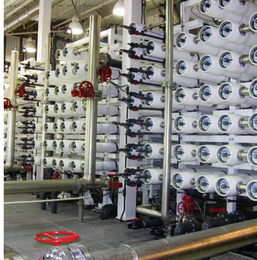
Mocho Groundwater Demineralization Plant
