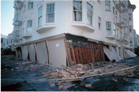
Damaged building due to lack of shear walls
