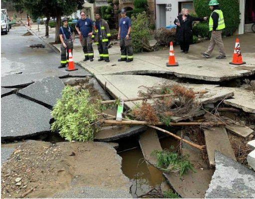
San Francisco Fire Department responds to water main break
