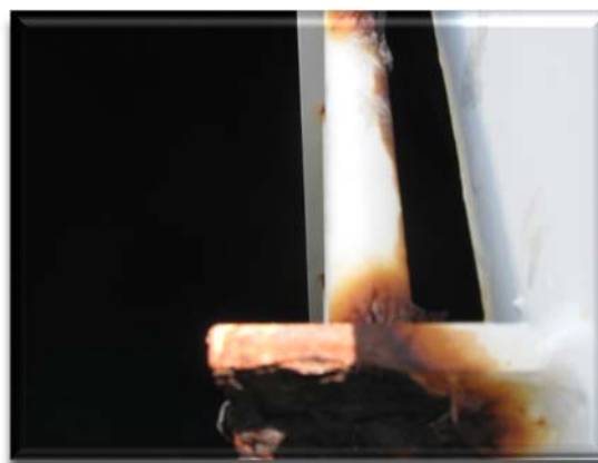
Difficult areas to prepare and coat have failed. The top of the ladder is an example of particularly poor condition.
