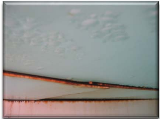
Seams between structural elements are also a typical failure point on the Dougherty Tank. This photo also indicates that blistering has developed on some broader surfaces.
