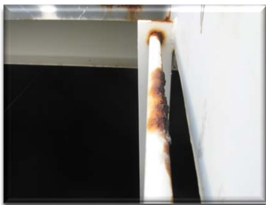
Ladder rungs have undergone significant corrosion where coatings have failed.
