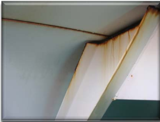
As is commonly the case, coating at edge and corner locations are failing.
